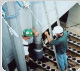
▶ Canada : water puri cation facility
