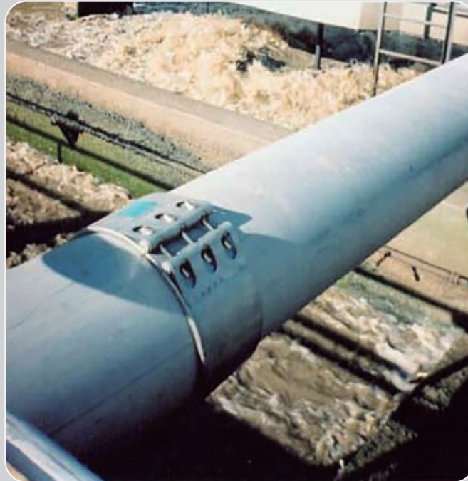
▶ Spain : water puri cation facilities
