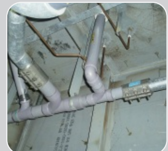
▶ PVC+Steel Pipe Connection
