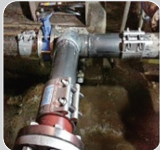
▶ Netherland desalination treatment facilities
